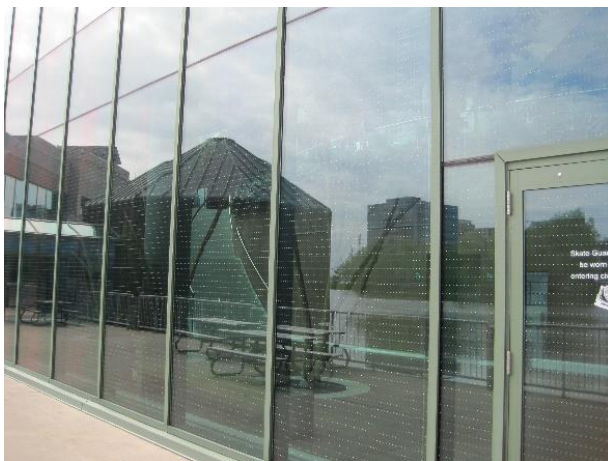
Figure 56. Feather Friendly at the Markham Civic Center, Markham, Ontario. Photo: Christine Sheppard
