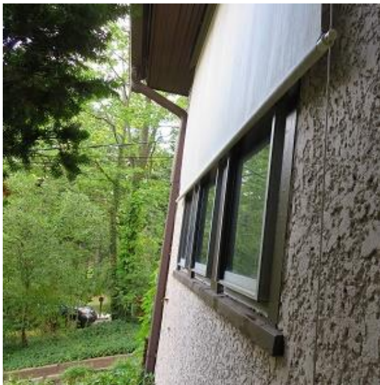
Figure 68. External motorized solar shades on a private residence. Photo: Christine Sheppard
